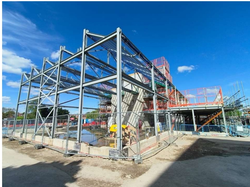
Sam Haile's shot of the completed steel frame in the April Sunshine
